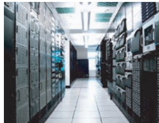
Collocation Space: A 120m special collocation space has been secured in the world’s largest data center. It flexibly responds to server expansions due to system enhancement.
